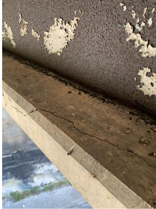
Photograph 7 – Localized crack in Beam B4 prestressed concrete encasement
