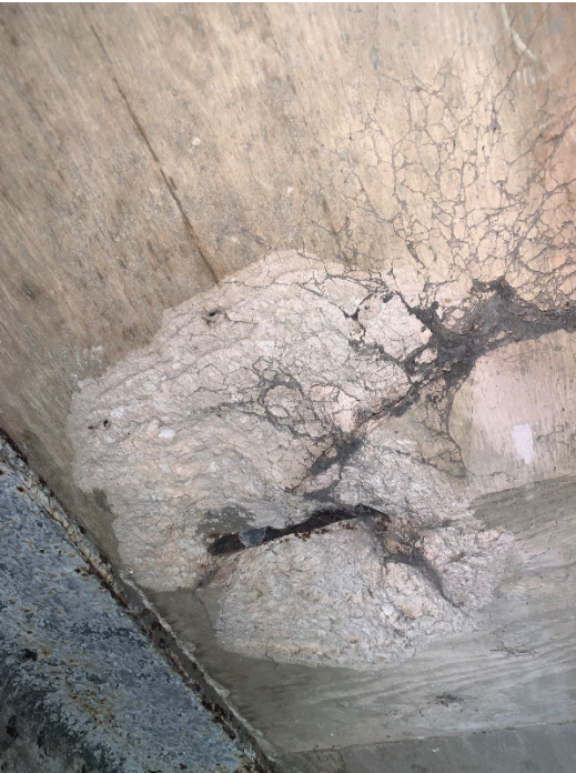
Photograph 14 – Example of localized spalling to bridge deck soffit
