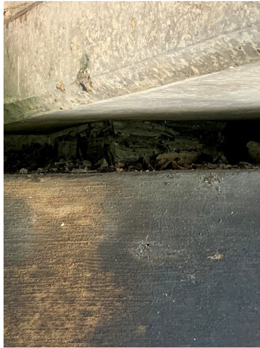
Photograph 11 – Example of severe corrosion of the bearings
