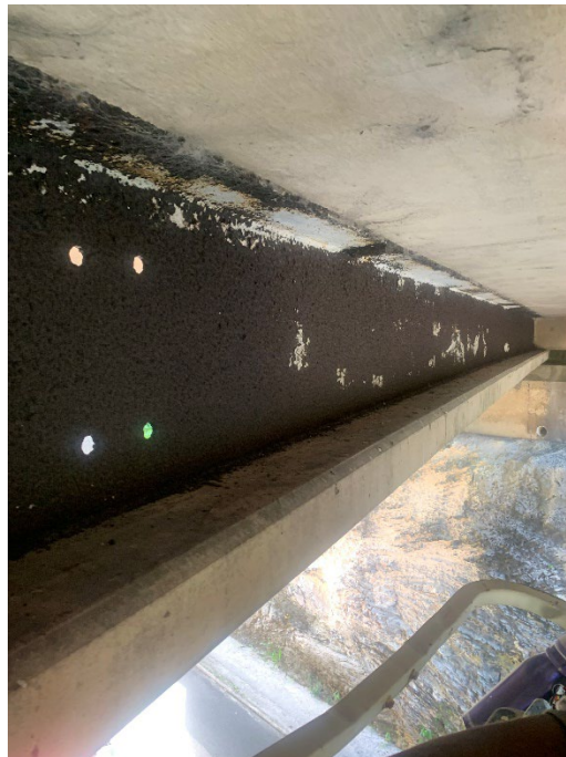
Photograph 2 – Example of the failed protective coating
