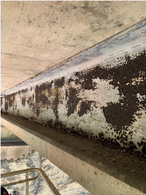
Photograph 3 – Example of the failed protective coating
