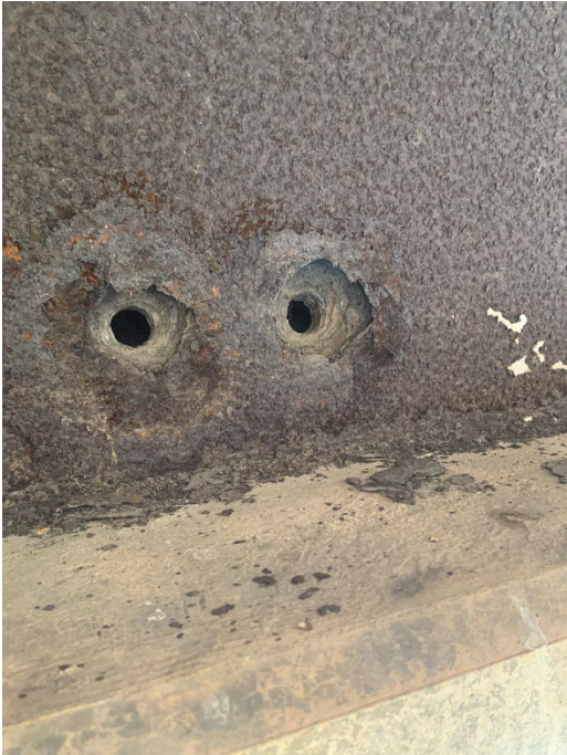
Photograph 4 – Corrosion of holes through Beam B1
