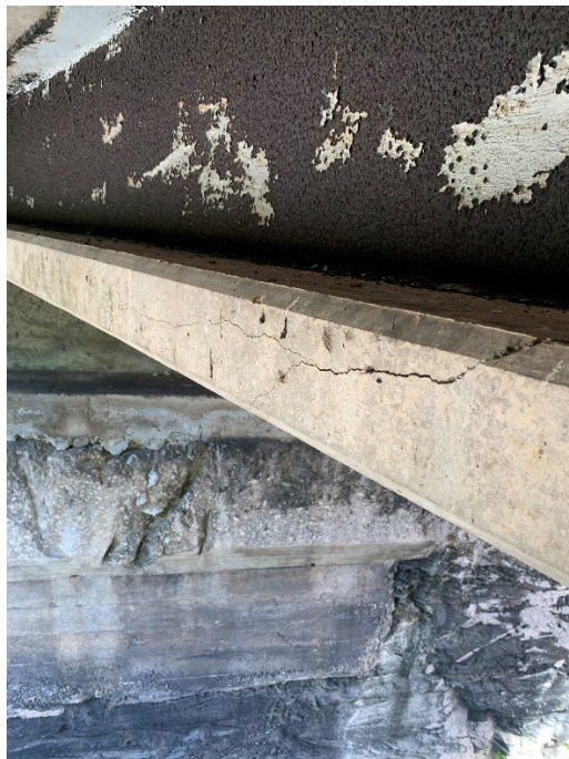
Photograph 8 – Localized crack in Beam B4 prestressed concrete encasement
