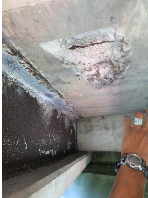
Photograph 15 – Example of localized spalling to bridge deck soffit
