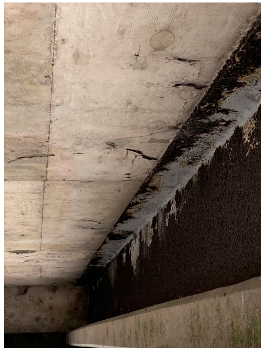
Photograph 16 – Example of localized spalling with concrete still attached to soffit
