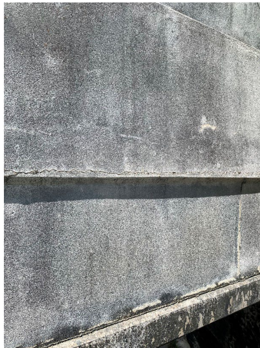
Photograph 18 – Crack along the eastern parapet
