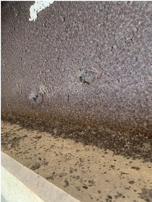
Photograph 10 – Localized evidence of corrosion pitting in Beam B7
