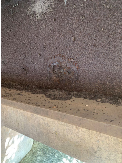
Photograph 9 – Localized evidence of corrosion pitting in Beam B7
