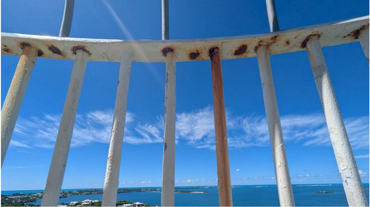
Photograph 15: Lower railings connection to intermediate rail in Section 4
