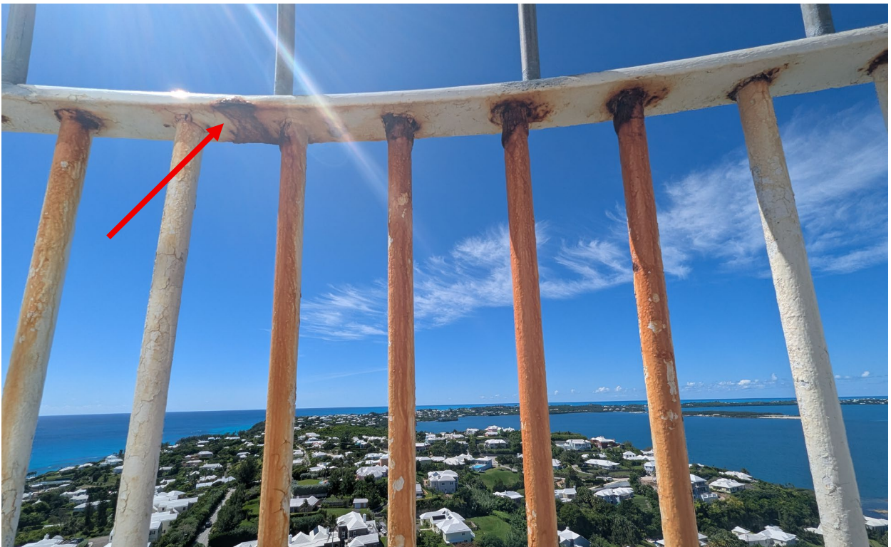
Photograph 18: Lower railings connection to intermediate rail in Section 5 (Bars 082-088) Intermediate top-rail between bars 86 to 87 exhibits corrosion
