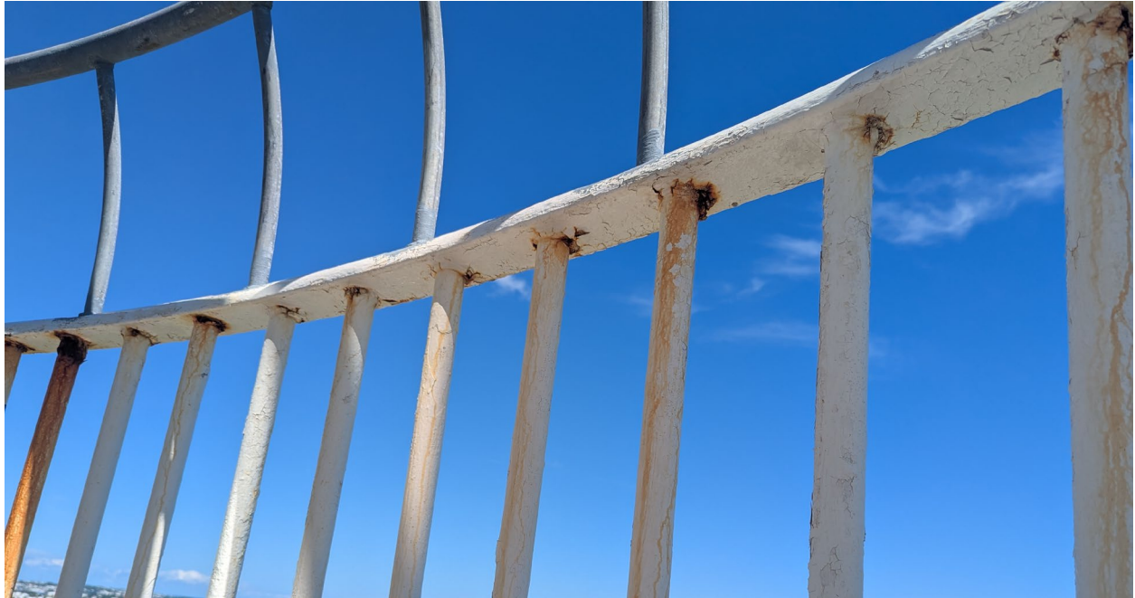
Photograph 7: Lower railings connection to intermediate rail (Section 1)
